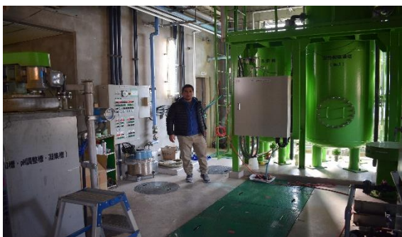
Chlorinator of a small wastewater treatment plant
