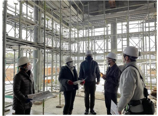
Figure 2: reflects training in Project Management & the use of PPP/PFI at the construction site of the Museum of Art
